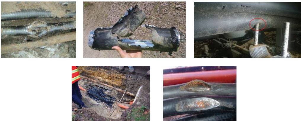
Fig. 4: Examples of mechanical failure resulting in short circuit fault
